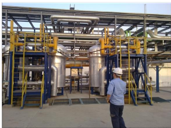
Purifier type TSA 34 000 Nm 3 /h – 10 barg (Air Liquide India)
