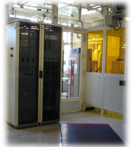
Oxygen purifier 10 Nm 3 /h – 8 barg
