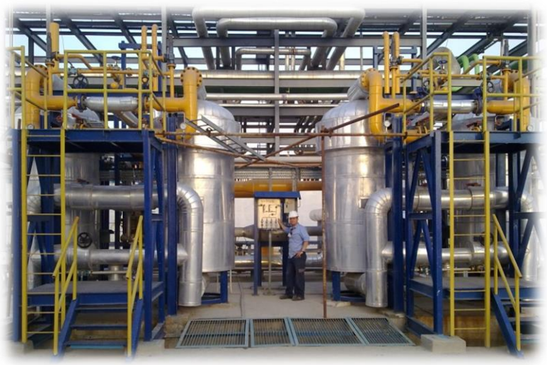
Nitrogen Dryer 34 000 Nm 3 /h - 8 barg
